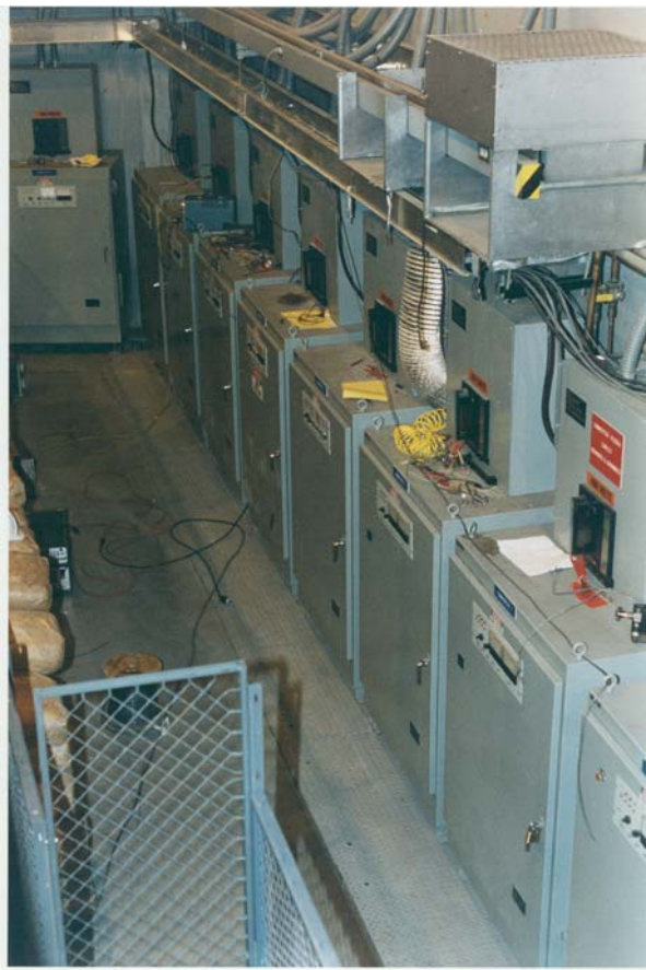
PTF Power Supplies
