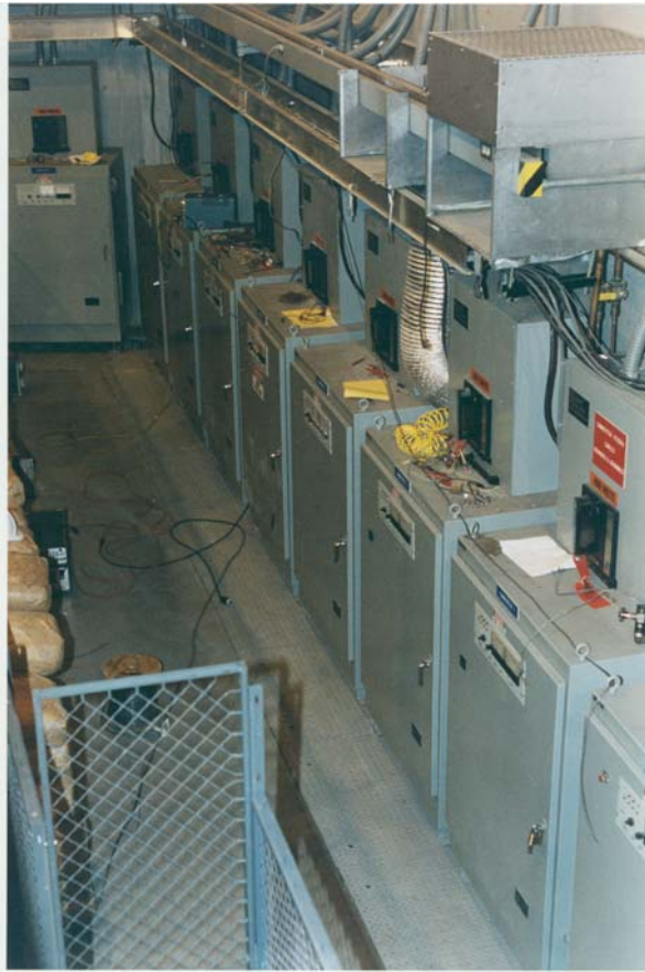
PTF Power Supplies
