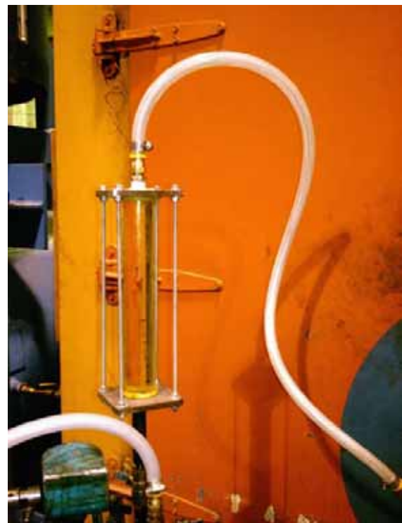
Epoxy fill site glass. Everson doesn't have a good method to measure the flow going into the coil
