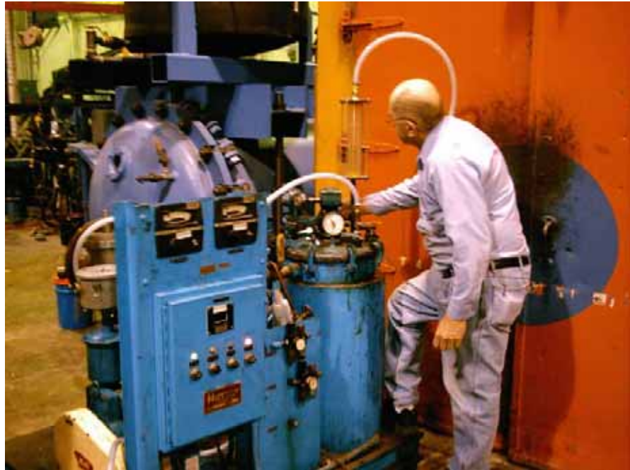
Lenny, an Everson Tech, watching the epoxy fill process A vacuum is maintained on the mold (inside the autoclave box) with a vacuum pump (not shown) to the right of the autoclave). The epoxy tank is at an atmosphere gage. Ron adjusts epoxy flow manually. After the mold is filled, pressure is cycled to drive off bubbles. The mold is under pressure during the cure cycle to minimize the remaining bubbles.
