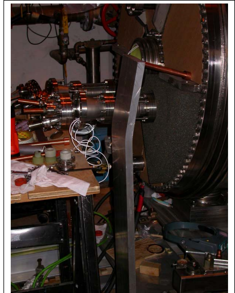
Bent Vertical Bus Bars have been received from Ramsey Welding
