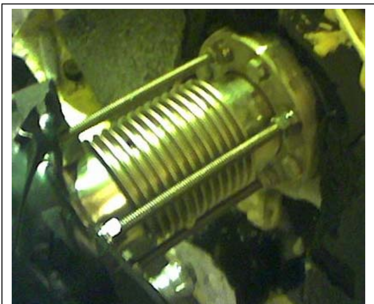
Leaks at the inner conflate of the terminal assembly appear to have been the result of the bellows tie rods not tightening the conflat
