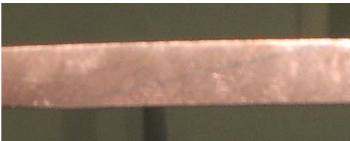
BNL Pulsed Magnet Manufacturing Status Sept 8 2004 Faint indication of silver soldered scarf joint
