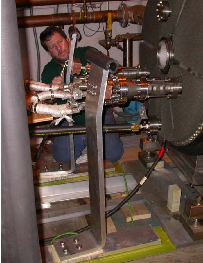
Magnet End of Bus Bars Silver Plated and Boltes
