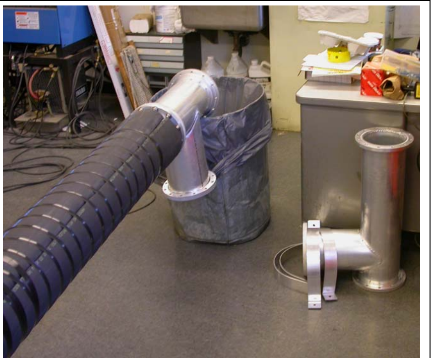
Insulated Vent Pipe
