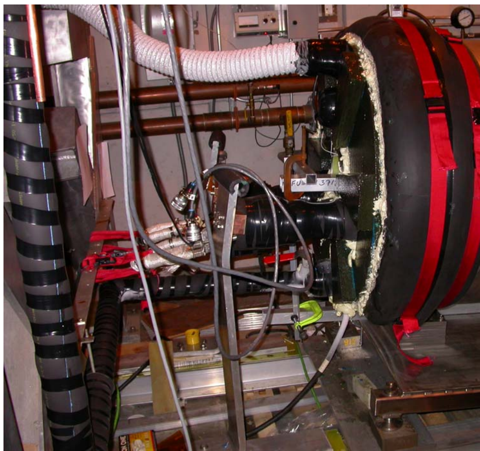
N2 gas duct is not insulated, and frosts up
