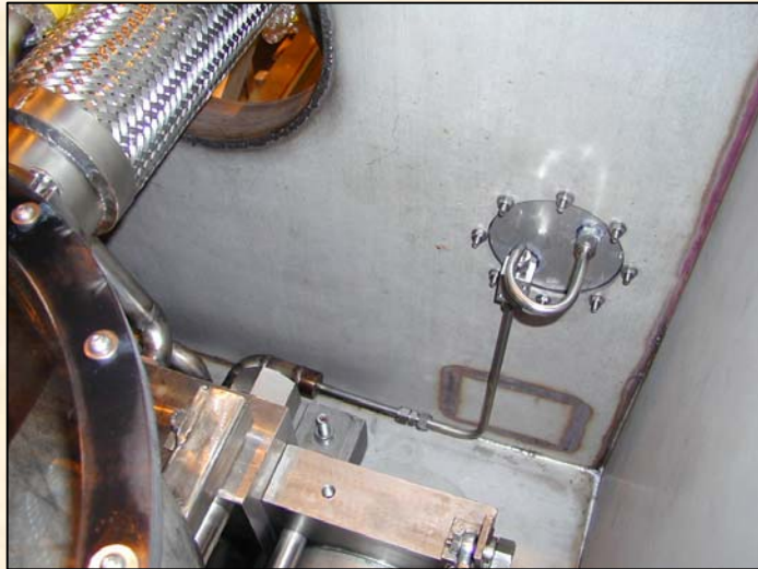
Hg drain from cylinder
