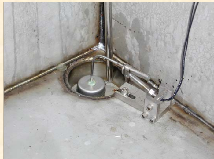
Hg leak sump with float switch
