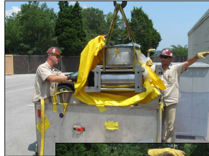
Mercury Cylinder & Sump
