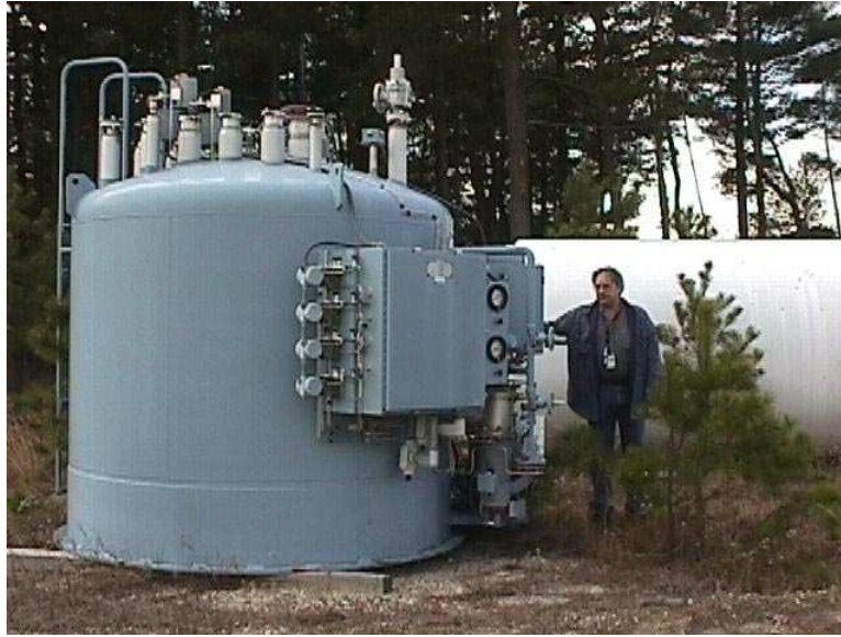
Figure 24: Photograph of the SSC-surplus heat exchanger (now at BNL) that is available for use in the proposed experiment.
