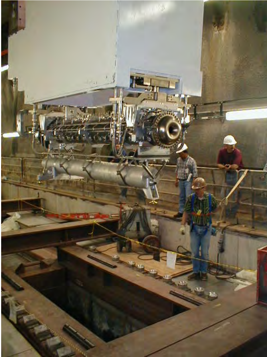
Figure 33: NuMI Horn 1 and positioning module installation in beamline chase.
